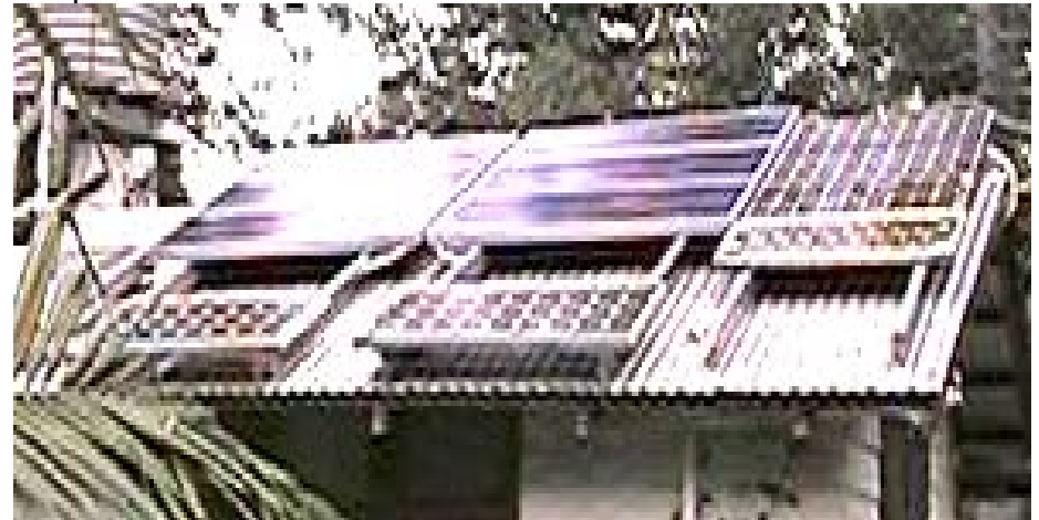
A number of panels in a system upgrade, installed on the roof of the bathroom.
